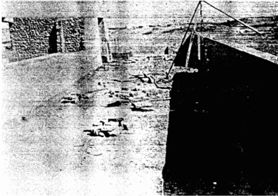
Photo 1: General view of the restoration works taken from the west showing the process of erecting the slabs at the southern wall.
